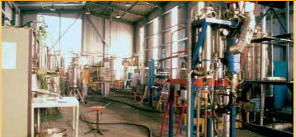
The industrial building at the INRA Laboratory for Food Processing Engineering and Technology, Villeneuve d'Ascq.
